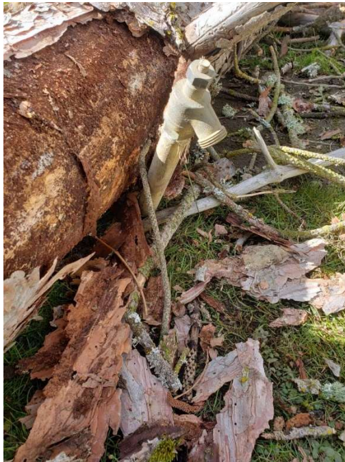
Figure 4 - Broken Water Spigots
